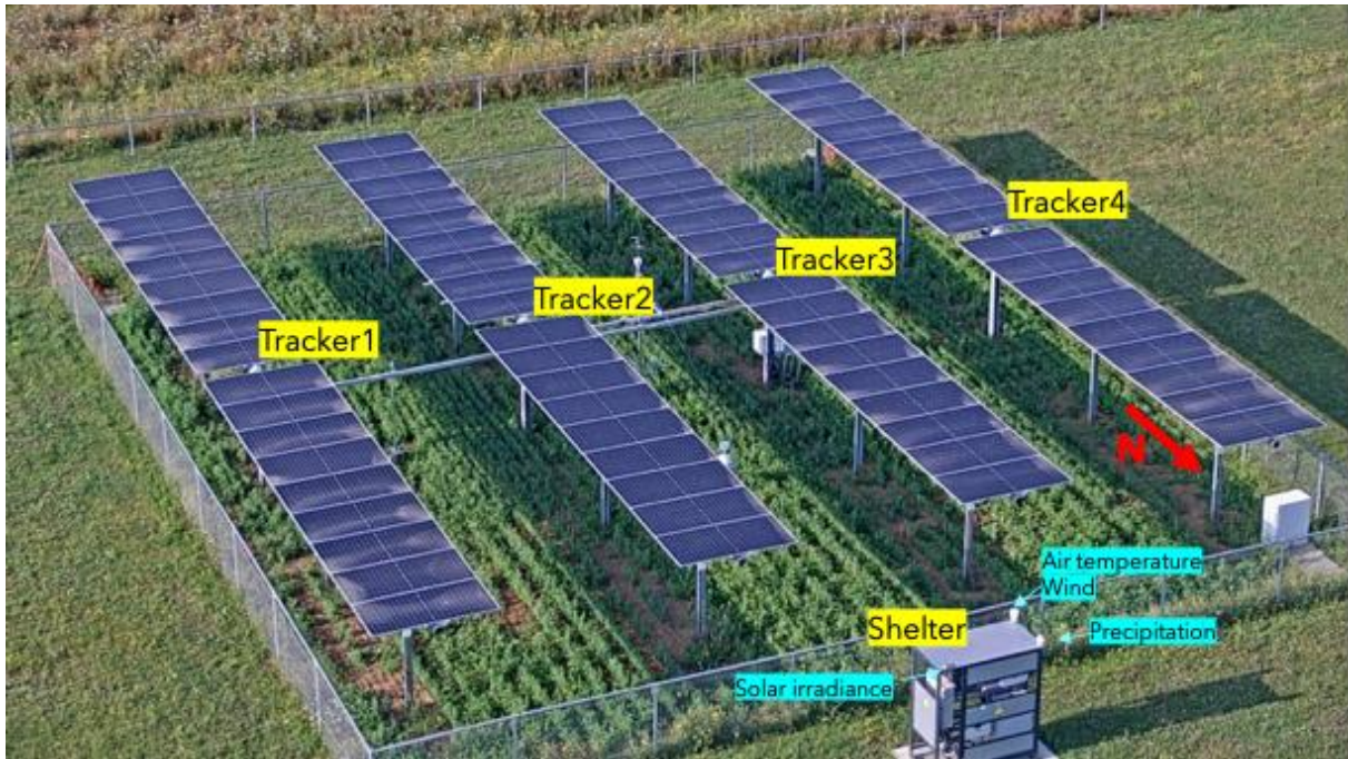
Figure 8 View of the tracking system elements and measurement sensors
