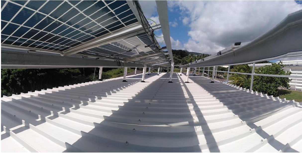
Figure 8 View of the ground under the PV modules (looking towards the East)
