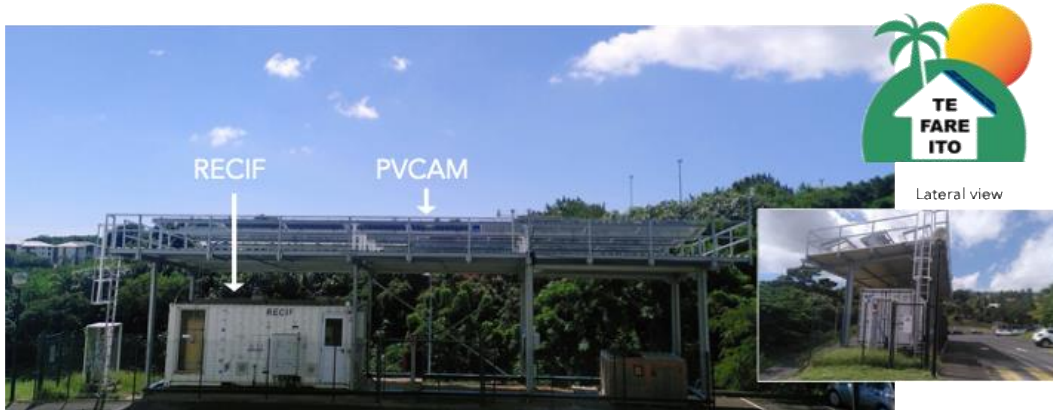
Figure 2 View of the Te Fare Ito installation, which hosts PVCAM and RECIF project platforms
