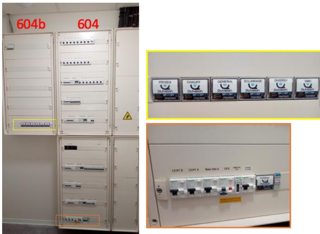
Figure 16 View of the 604 electric panel after having installed 7 Spooky devices in two zones that are zoomed-in on the right. The orange zone contains a Spooky that allows to open/close the water heater circuit remotely.
