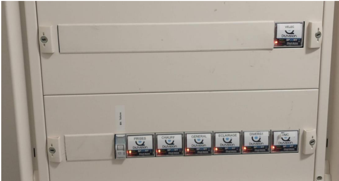
Figure 18 View of the 604 electric panel after having added the Spoony to count the exchanges with the Vehicle2Home charging station
