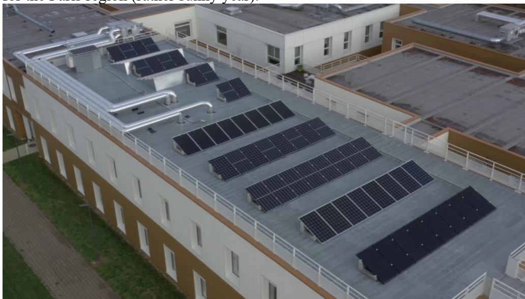
Figure 5 View of the Drahi-X photovoltaic roof-top installation
