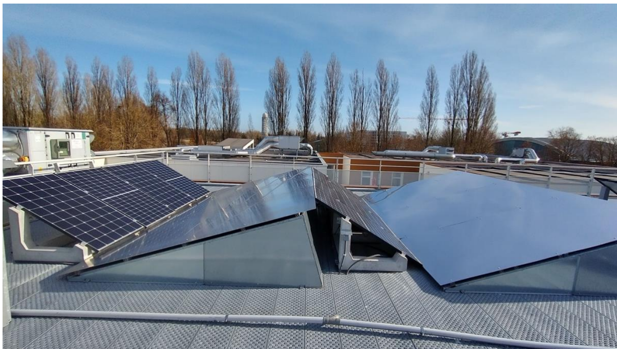
Figure 4 View of reflectors installed for panels #45 to #52. The installation of these reflectors were done between the 26 Oct 2021. This installation implied the shift of panels #43 and #44 about 30 cm to the South and it implied that, from then on, these two panels suffer a bit more from shading in winter (from the front row, that is panels #41 and #42).
