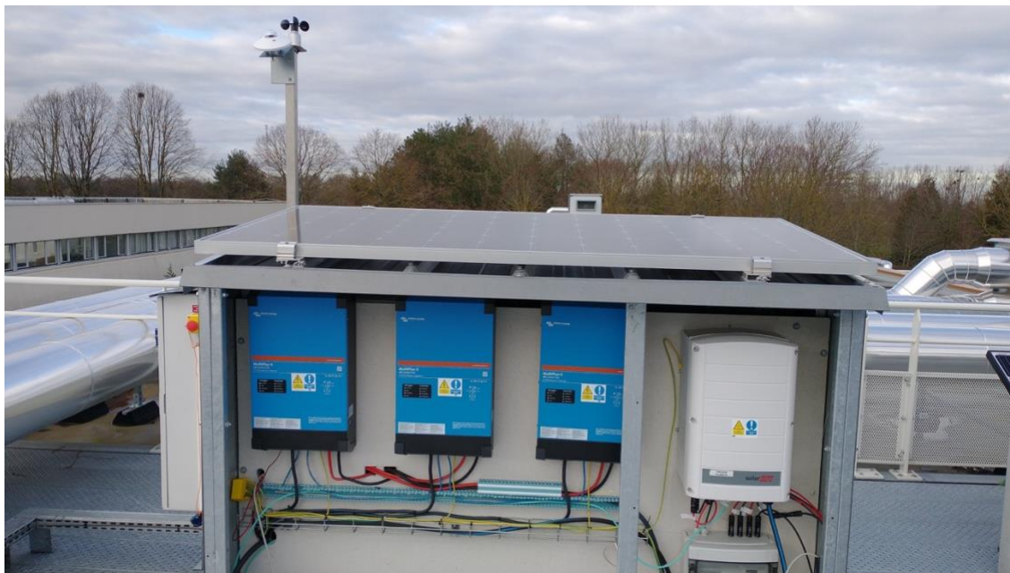
Figure 9 View of the battery (in blue) and PV (in blanc) inverters on the roof of the Drahi-X building
