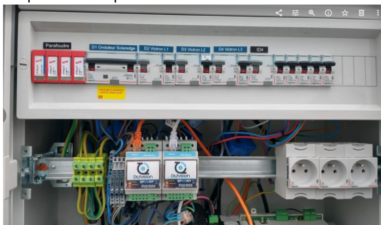
Figure 17 View of the electric panel on the roof of the Drahi-X building after having installed two spookey devices in order to count the photovoltaic and battery electricity.
