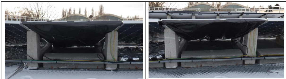
Figure 25 Panels #36 (left) and #38 (right) were covered with a black plastic on the rear side for one year (4 Feb 2021 to 18 Mar 2022) as an experiment to estimate the bifacial gain of the panels (by comparison).
