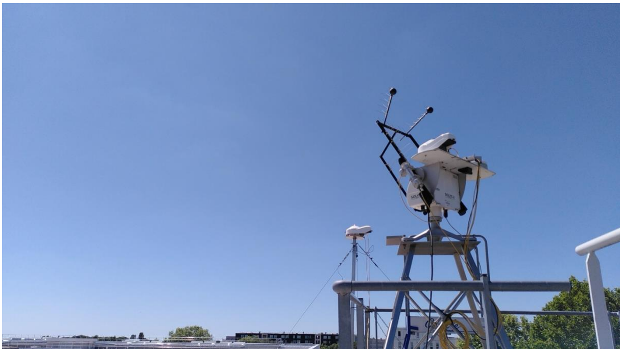
Figure 5 BSRN (baseline surface radiation network) installation at SIRTA with Global, direct, diffuse solar irradiance as well as infrared irradiance measurements
