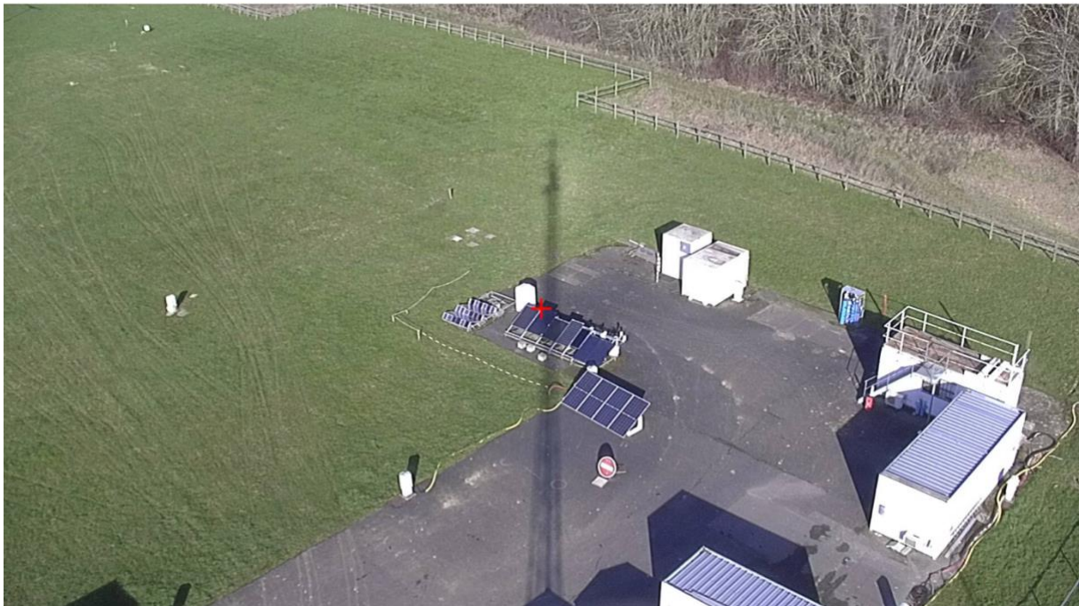
Figure 3 View of SIRTAs PV installation at the beginning of 2022 from the camera on that 30 m mast. The photo also shows the shading impact of this mast on PV1 installation.
