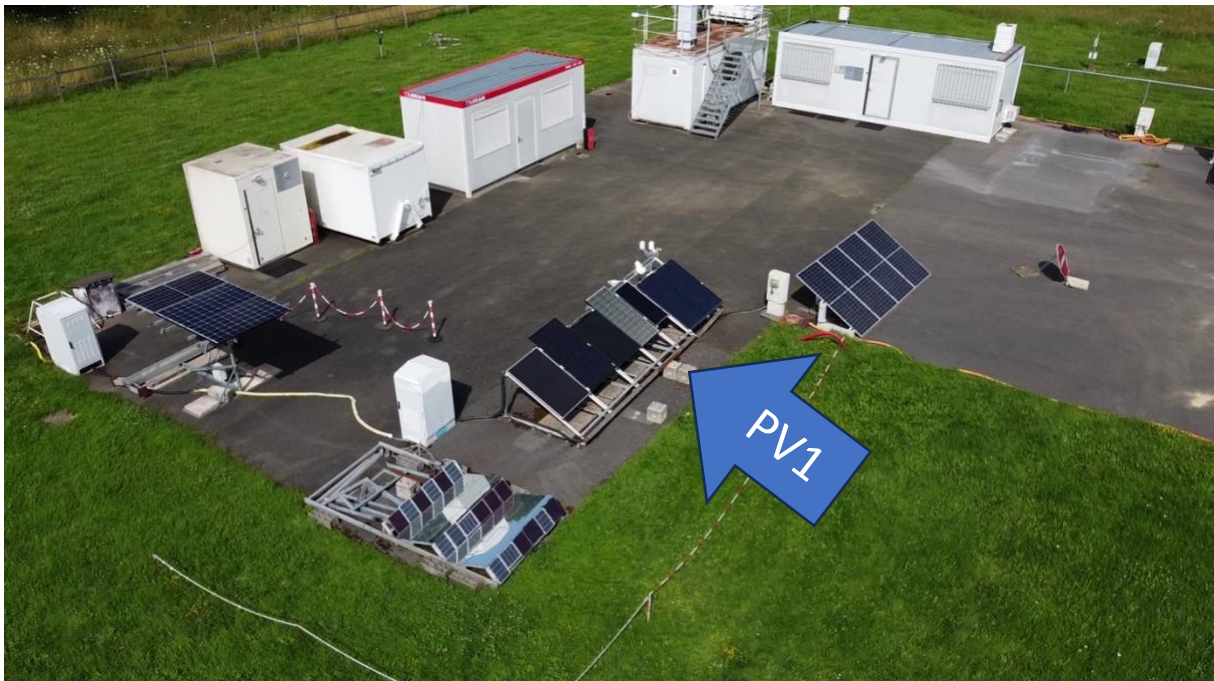
Figure 4 Drone's view (from the South-West) of SIRTAs PV platforms in July 2021
